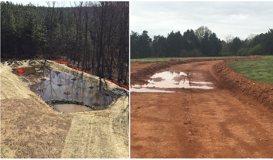
Figure 7. Example of compliance (left) and noncompliance (right) with erosion and sediment control requirements. Photos courtesy Berkley Group.
