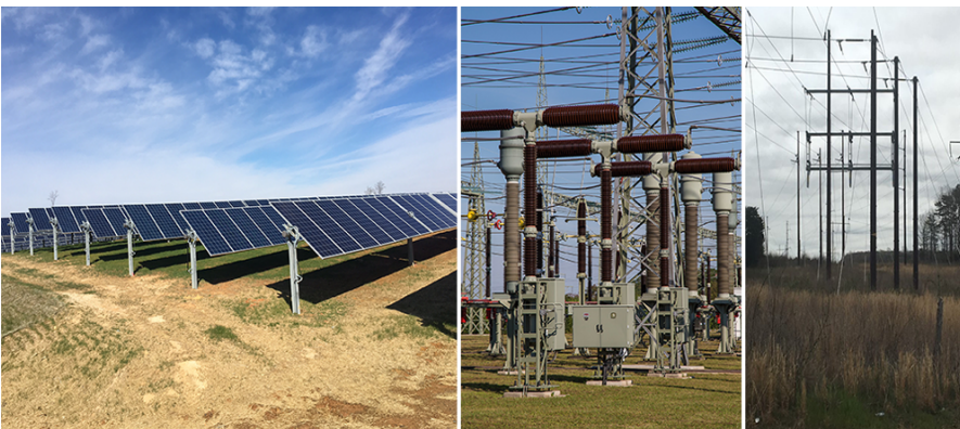
Figure 2. Components of a solar farm: solar panels (left), substation (center), and high-voltage transmission lines (right). Photos courtesy Berkley Group (left, right) and Pixabay (center).
